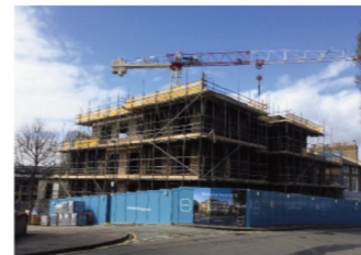
Marischal Road, SE13 26 Pocket Homes Prices TBC Completion in Winter 2016 Achieved unanimous consent
